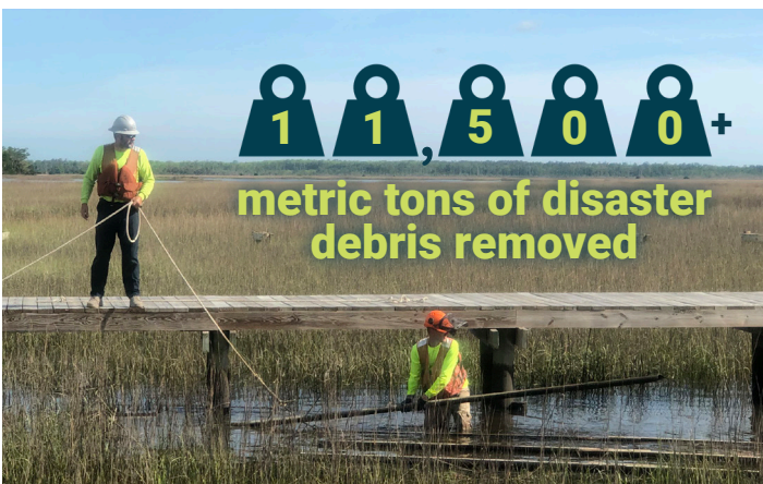
Contractors work to remove several hundred feet of wooden dock debris from the marsh in Glynn County, Georgia (Photo: NOAA).
